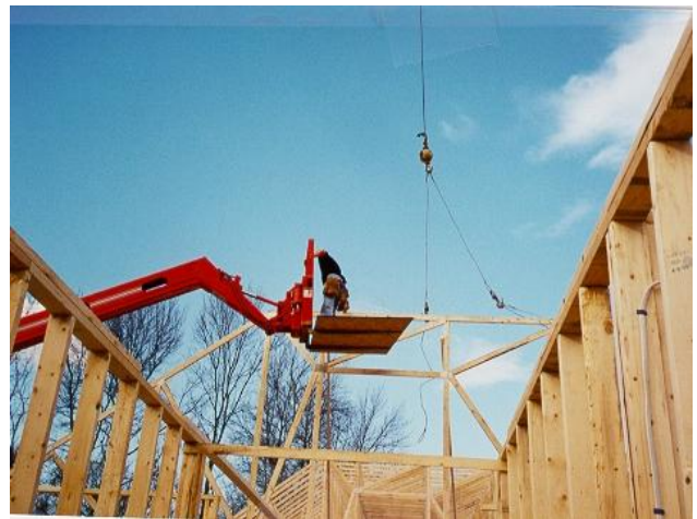
Lifting employees on the forks is unsafe and unacceptable!
