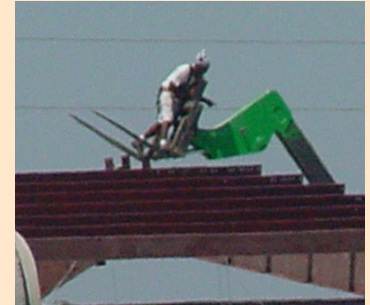
There is no platform or fall arrest system used in this photo.
