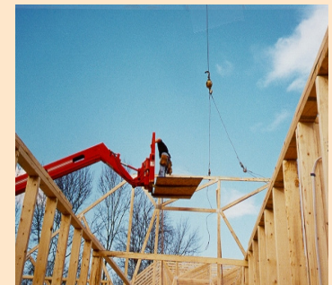
There is no guardrail or fall arrest system used in this photo.
