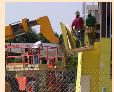
This is an improper platform and there is no fall arrest system being used.
