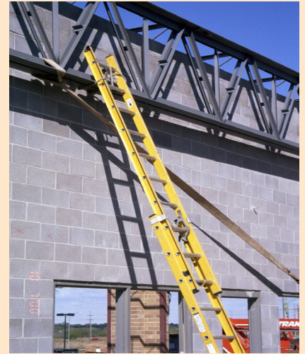
This is an example of ladder securement.
