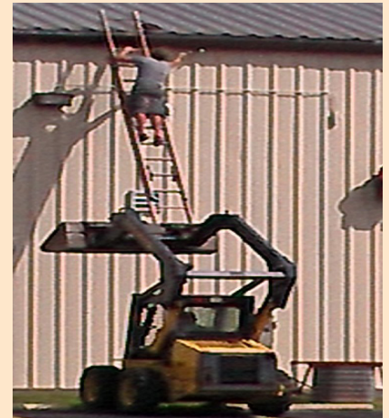
This is a poor example of how to secure a ladder.
