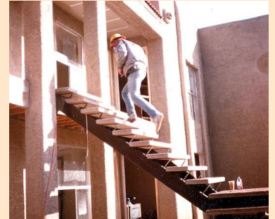
Without the use of guardrails, employees could easily fall.
