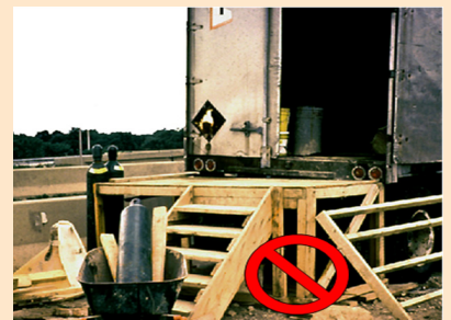
The stairway to this platform has more than four risers and needs guarding.
