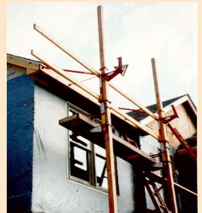
Incorrect: The ends are not guarded.
