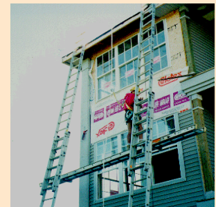
Correct: Safe access is provided and the employee is wearing a fall arrest system.
