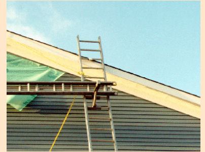
Incorrect: Safe access is not provided to the work platform.
