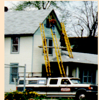
Unsafe: Ladder feet not stable on a sloped roof.
