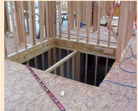
Large openings require guardrails. Use toe boards if tools could fall on employees below.
