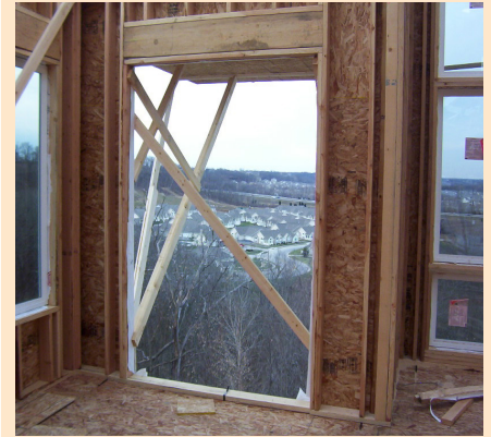
Set up guardrails if employees could fall through a window, door or dormer openings.
